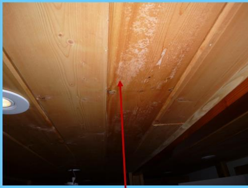
Visible damage to wood ceiling finish. Also some cupping and shifting of ceiling noted.
