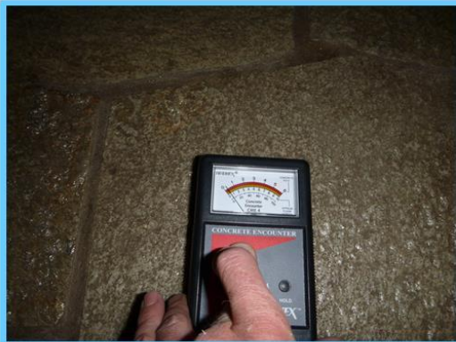
Electronic non penetrating moisture reads about 2% at the unaffected entry taken from multiple readings.
