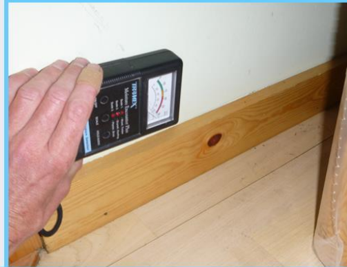
Moisture readings are over 30% with furniture, baseboard, drywall, and flooring remaining.
