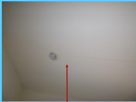
Moisture stains from around light fixture.
