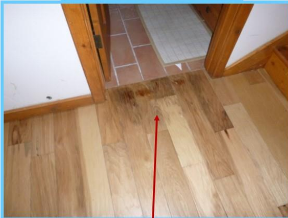
Water staining on wood floor.
