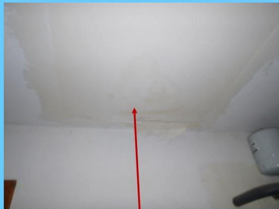
Moisture damage to ceiling at south corner under bathroom.
