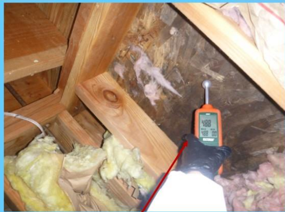
Slightly elevated moisture.
