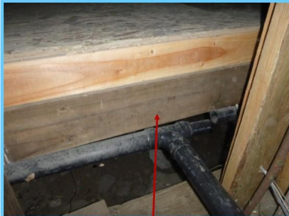
Framed platform obstructs access to entire crawlspace.
