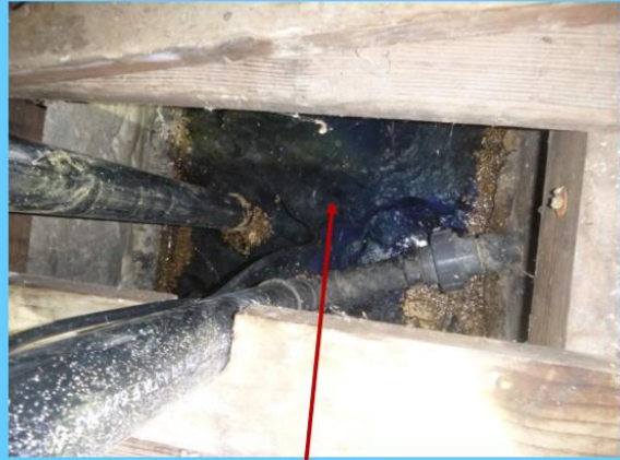
Contaminated water in pit.
