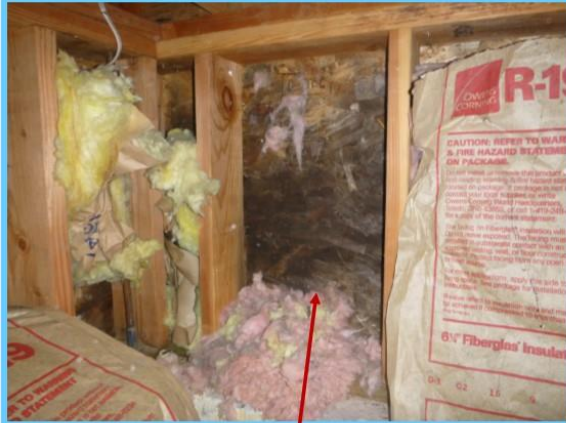
Atypical mold on the perimeter wall.
