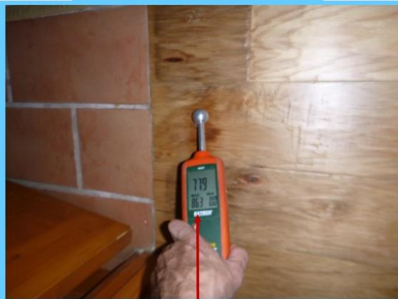
Elevated moisture in flooring.
