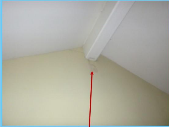
Moisture damage to wall surface over ridge beam hanger.
