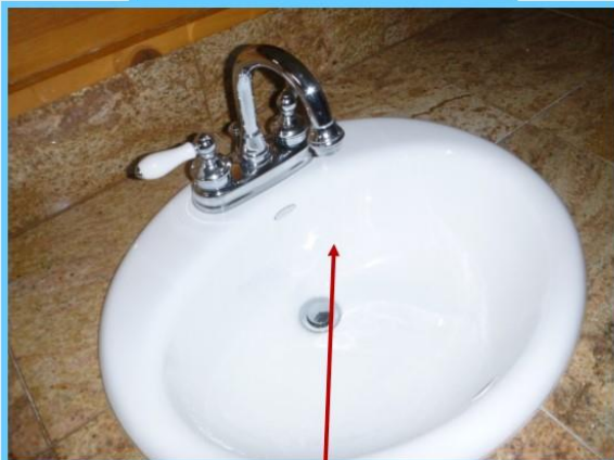
Faucet is dripping.
